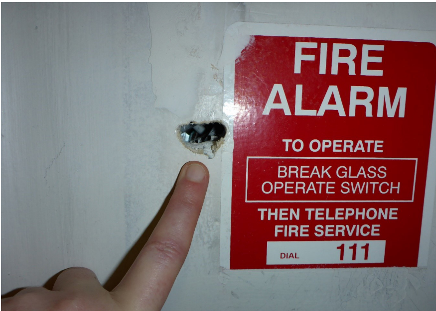
Hole in compartment wall
